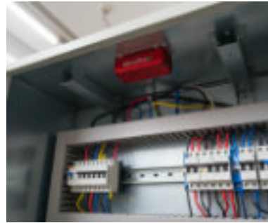
Electrical cabinets, cable ducts, and meter boxes
