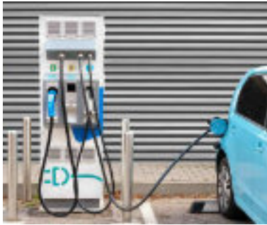
EV and Charging stations
